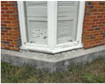
Sample of Needed Window Frame Repair
