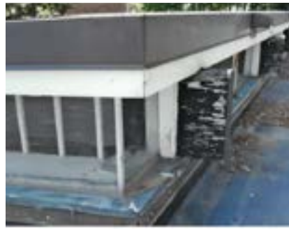
Beam Ends Before GBP
