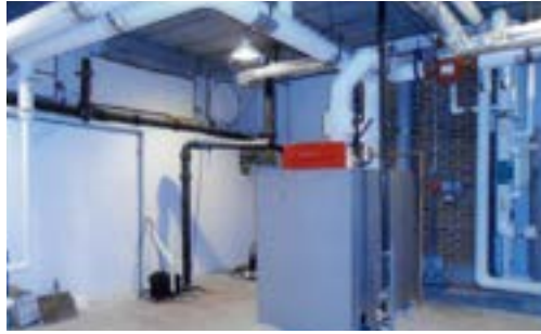
Furnace Room After GBP
